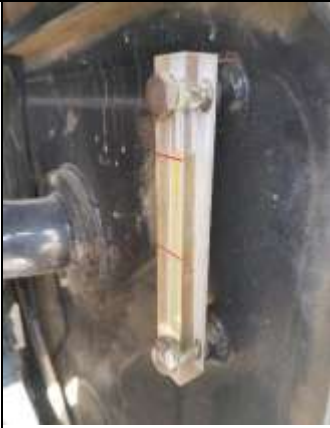
Hydraulic level gauge found satisfactory at the time of inspection
